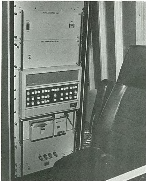
Figure 2-34. Automatic Train Control Equipment Rack
